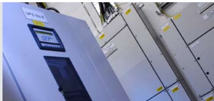
■ 100kVA Master Plus UPS powering the air conditioning system
