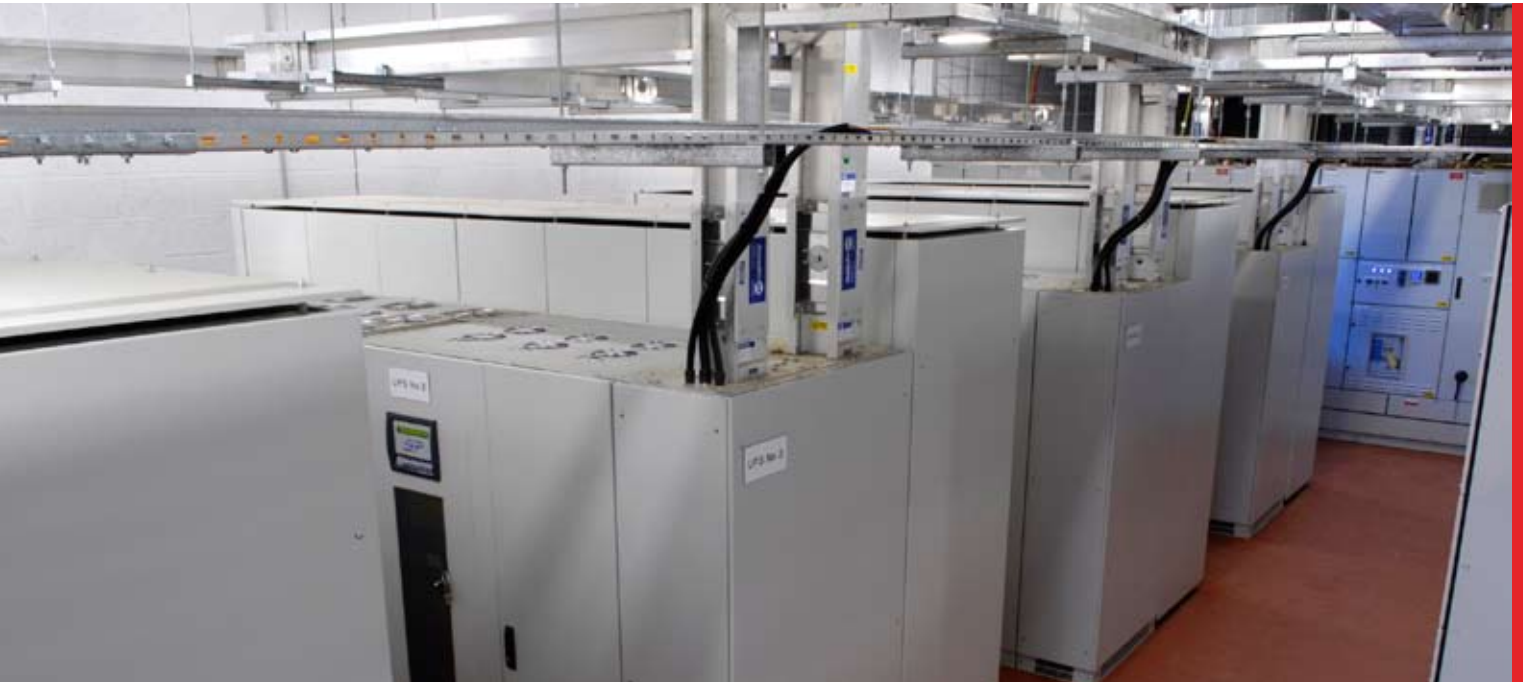
■ Plant Room showing the 800kVA Master Plus UPS with side cabinets and top entry Barduct
